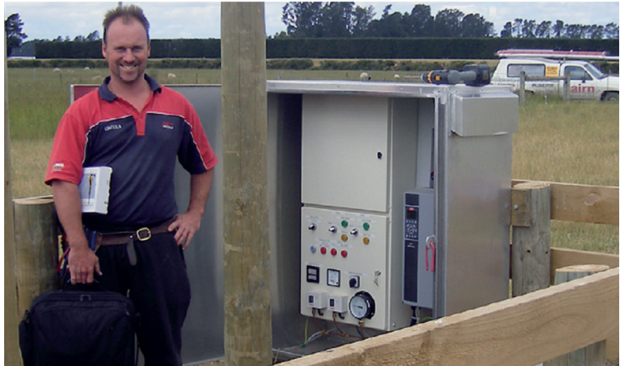
Lincoln Teale in front of one of Nairn Electrical's irrigation pump control solutions.
