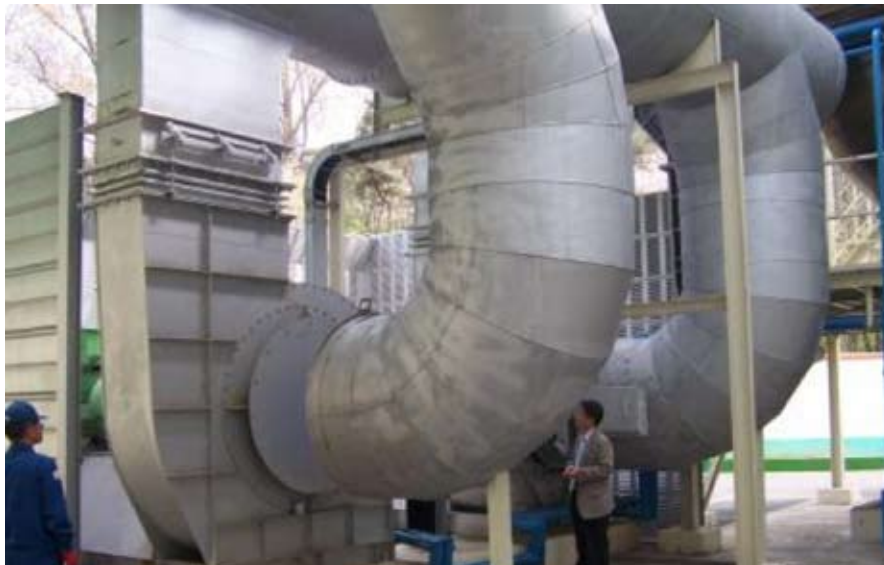
The ID fans in the Korean incinerator plant
